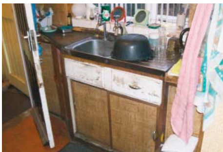
A kitchen older than 20 years that will be replaced as part of the programme.
