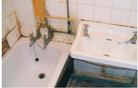
A bathroom older than 30 years that will be replaced as part of the programme.
